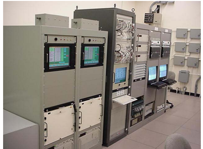
Figure 5. The operations room at Lorsta George, WA
